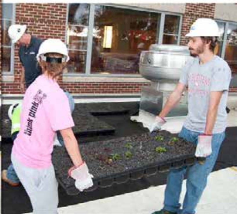
Dr. Richard A. Niesenbaum (left) and his students (top and bottom right) installing the green roof on the Wood Dining Commons
